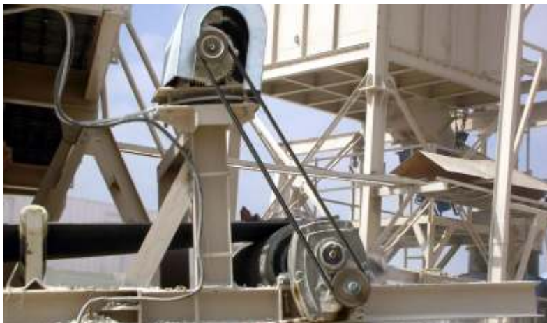
Conveyor Application in a Stone Crusher Plant
